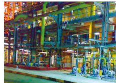
FERRIC CHLORIDE PLANT EGYPT
