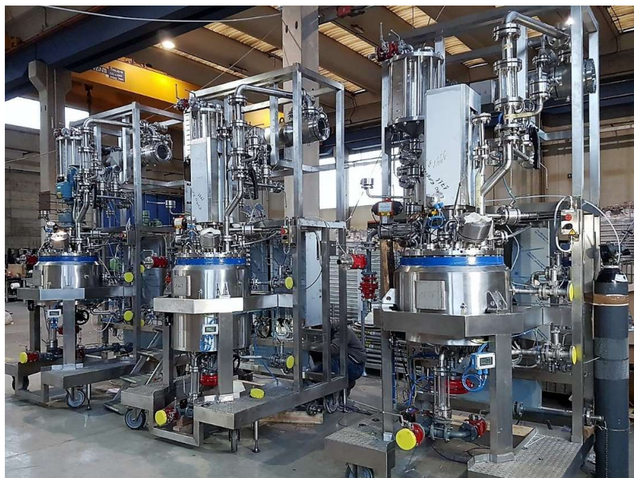
Complete Reactor System
